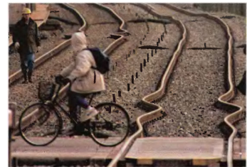
FIGURE 15.14 Thermal expansion. The extreme heat of a July day in Asbury Park, New Jersey, caused the buckling of these railroad tracks. (Wide World Photos)
